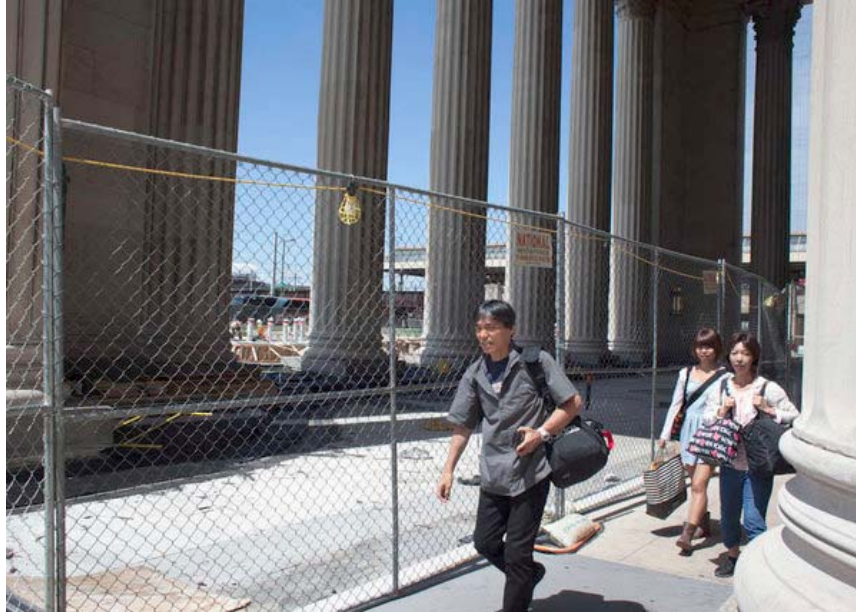
Construction on the west end of Amtrak's 30th Street Station continues, but the arrival of the $60 million funding from Congress for the planned exterior restoration of the limestone facade of the 80-year-old neoclassical building is unclear. (ED HILLE / Staff Photographer)
